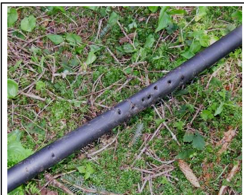
Bear damage to the water system hose
